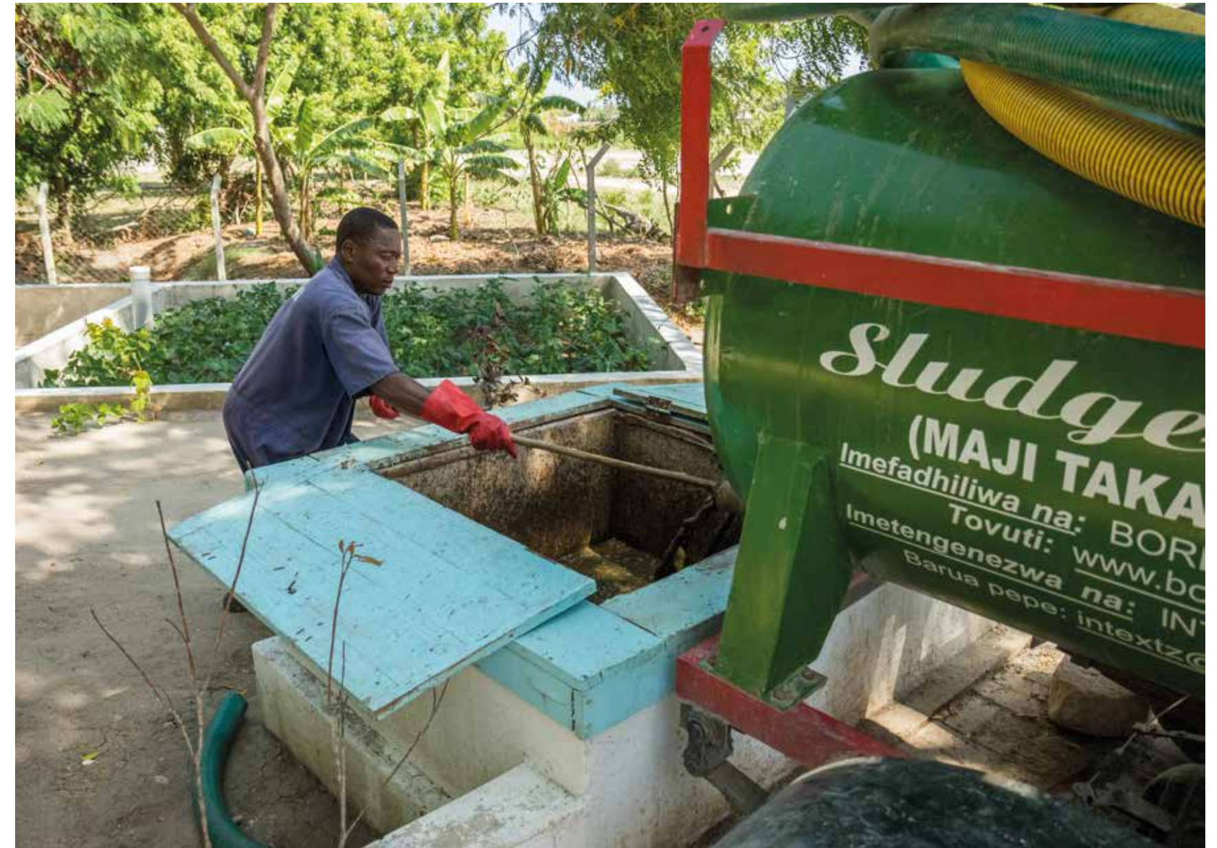
Kigamboni treatment plant →
